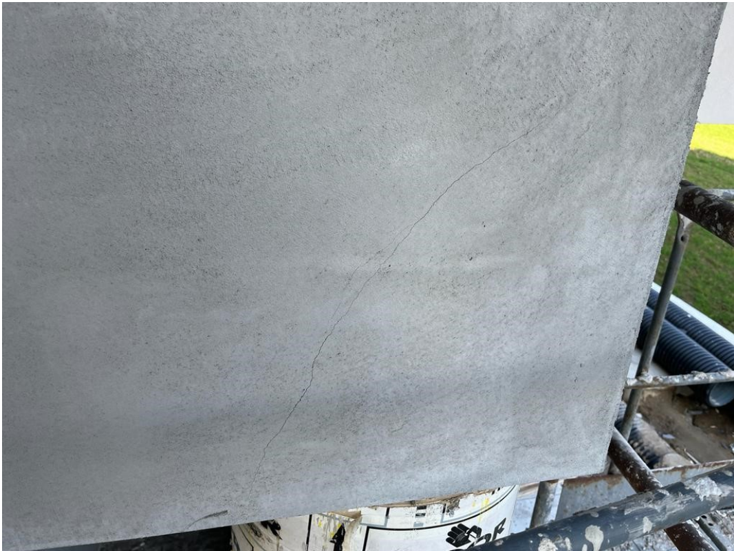
Excessive thickness of cement-based render
