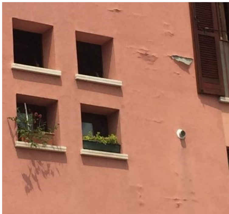
Total detachment finishing coat from reinforced skim coat
