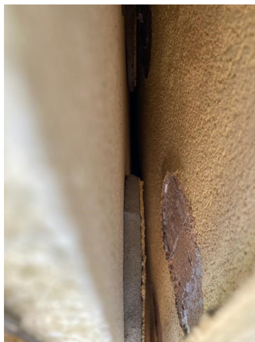
Detachment of the old finish coating
