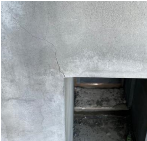
Failure or misplacement of diagonal mesh patches
