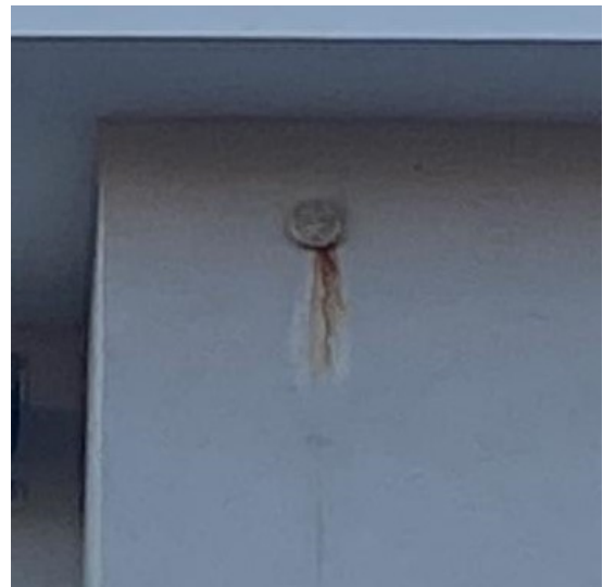
Failure to place the sealing tapes
