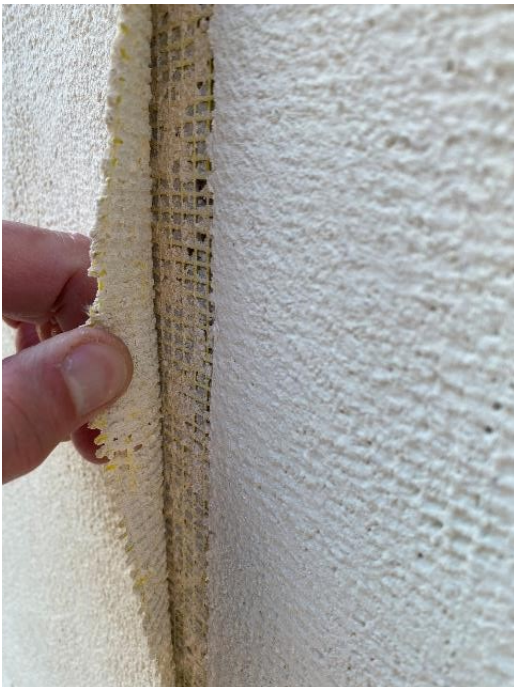
Misplaced mesh and insufficient thickness of the render
