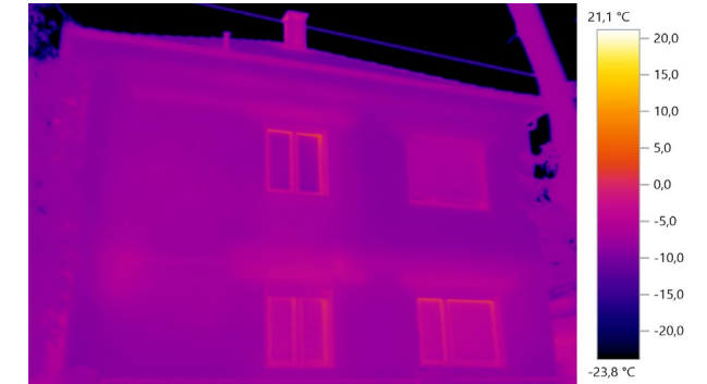
Scale is set too high: It appears that no renovation work is required
